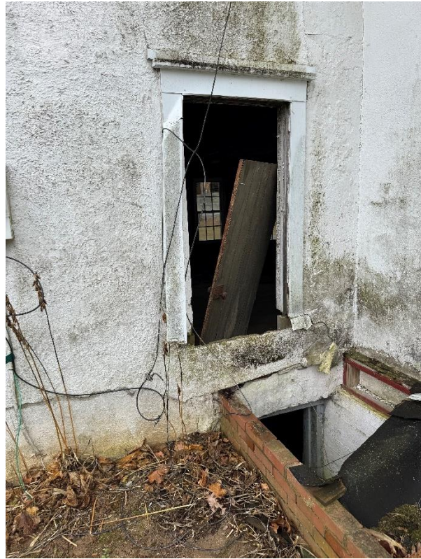
MISSING REAR DOOR AND OPEN BASEMENT
