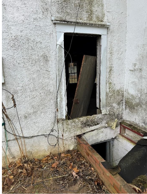
MISSING REAR DOOR AND OPEN BASEMENT
