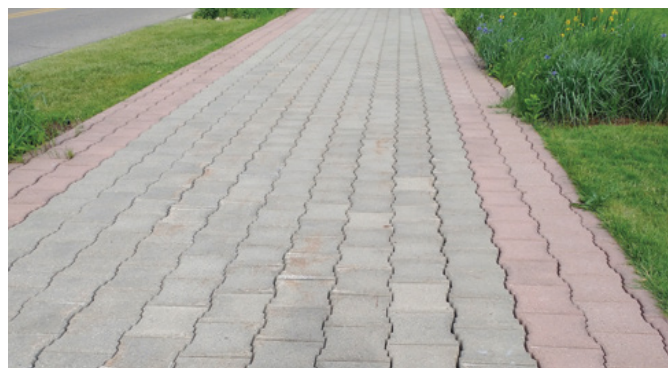
Figure 29a. Permeable block pavers infiltrate runoff before it flows onto the lawn or street. (Andy Yencha)
